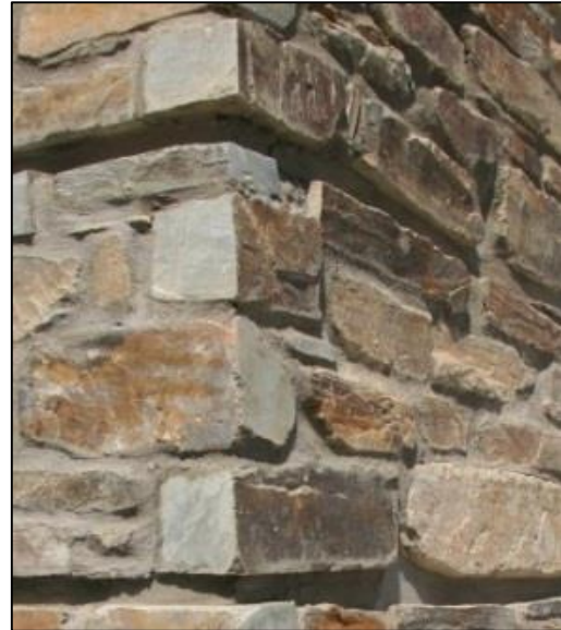
'Cut quoins' from other 'rustic stone' supplier (Lantoom Quarry).
